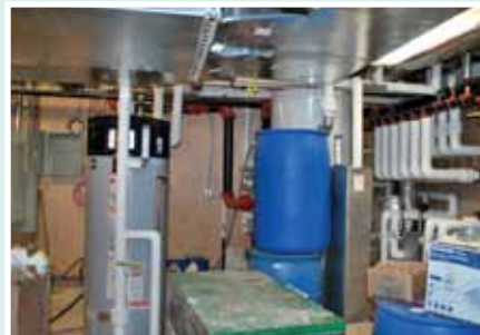
The mechanical room in the residence, where equipment for the geothermal heating and cooling system, water filtration, sprinklers, and hot water production resides.
